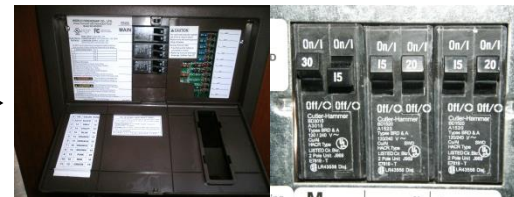
Fuse box with Circuit Breakers
